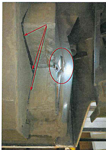
Image 20: Right portal side of threshold doorway #4- broken welding seams
